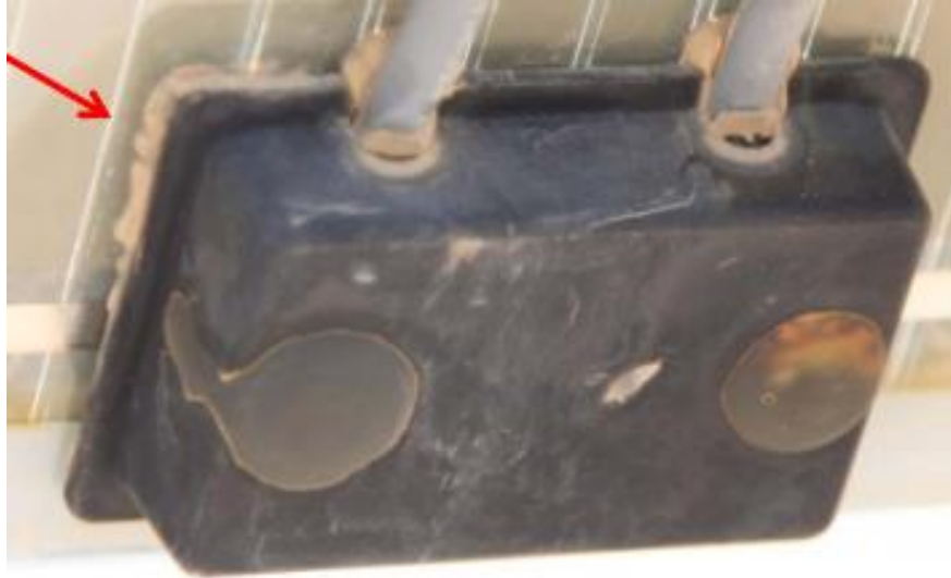
Figura 7.31. Junction Box desprendida 11
